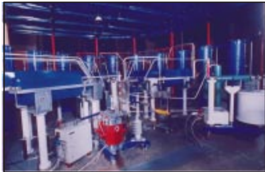
Impulse Current Generator 100 kV, 150 kJ
