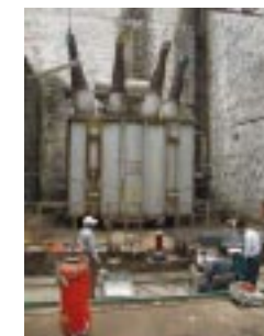
Diagnostic testing of Power Transformer
