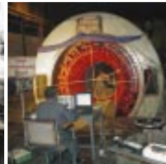
ELCID Test on Turbo Generator Stator Core
