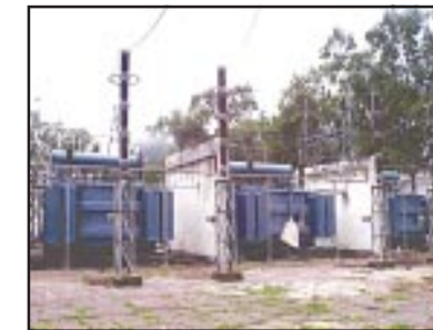
Test Setup for Switching test on OLTC
