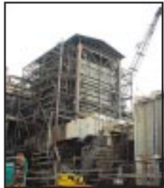
Coal fired boiler – 210 MW
