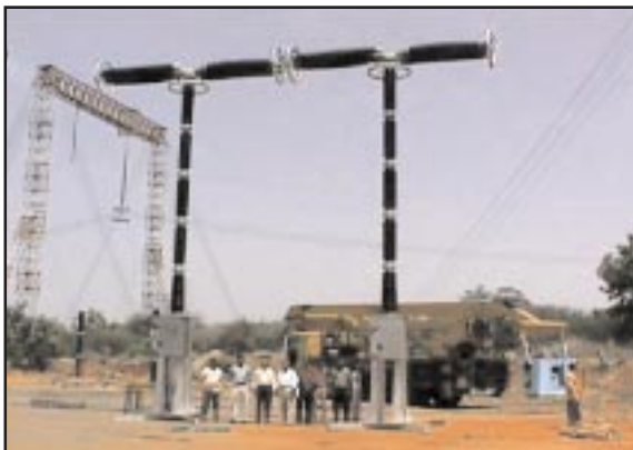
800 kV Circuit Breaker erected for testing
