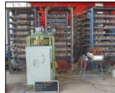
132kV Switch Yard of Station - II
