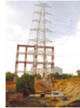
400 kV M/C type 'QA' tower
