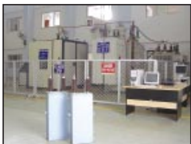
6800 KVA, 50 kV Resonance Test System
