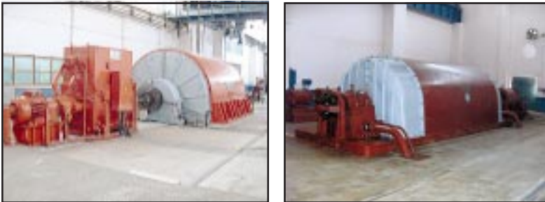
View of Short Circuit Generators
