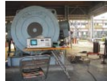
Diagnostic testing of HV Motor
