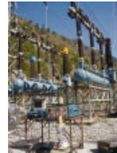
Diagnostic Testing of Sub-station equipment
